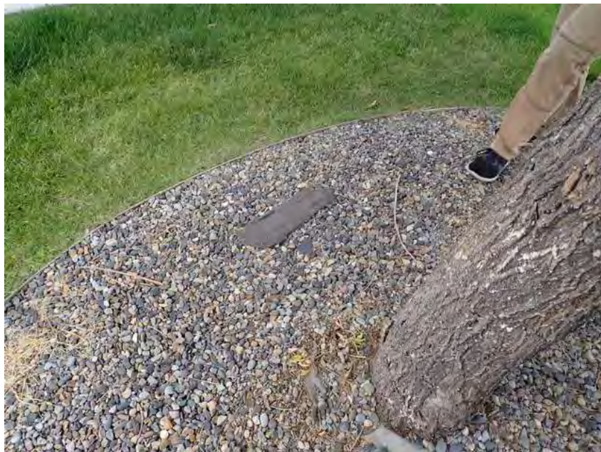
96. Building 6 Found portion of shingle on ground.
