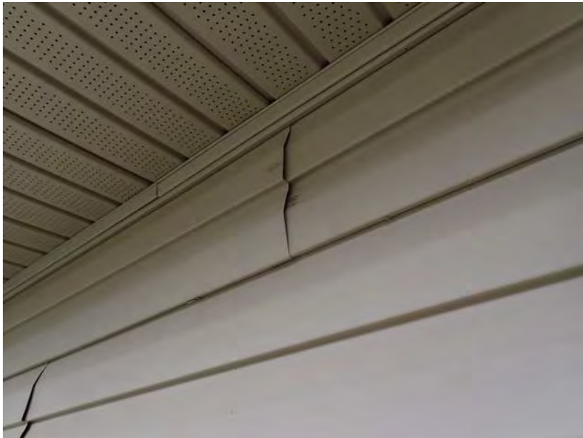
76. Building 5. Gap in siding likely due to installation issues.
