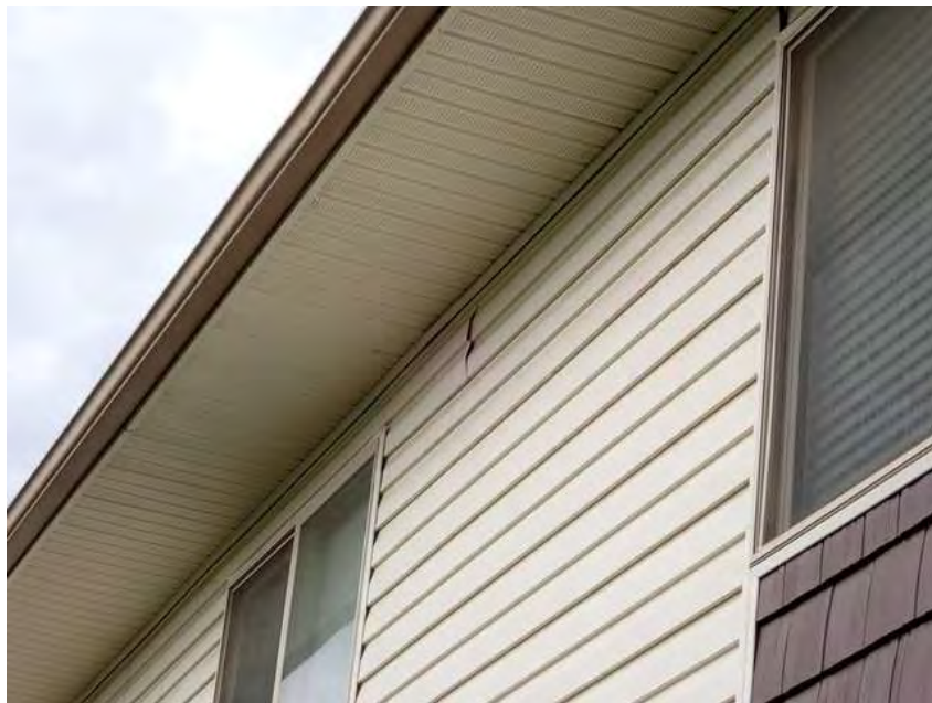
48. Building 3. Gap in siding.
