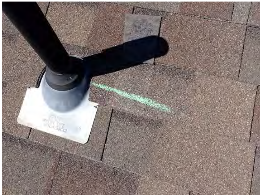
382. Building 22. Creased tooth on shingle.
