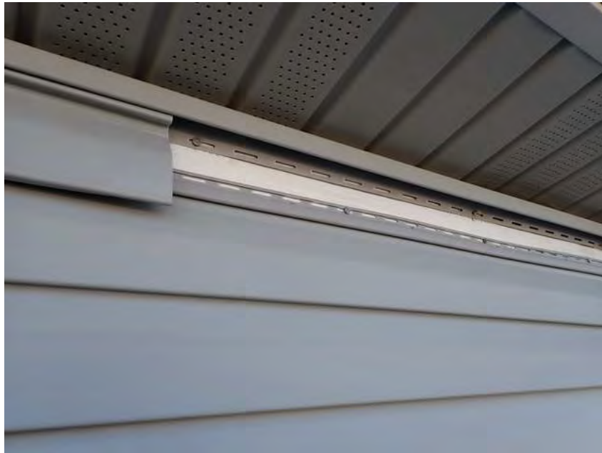
349. Building 20. Missing siding.
