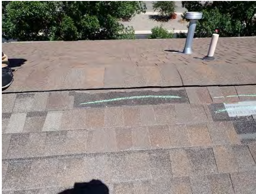
117. Building 6 missing shingle from recent winds.
