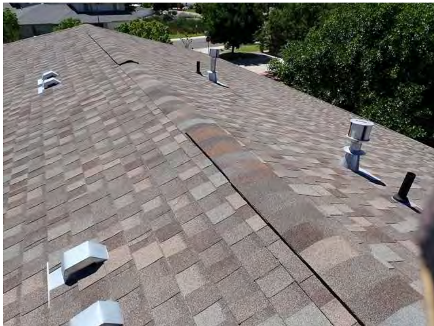
54. Building 3. Possible mismatch on ridge cap shingles.
