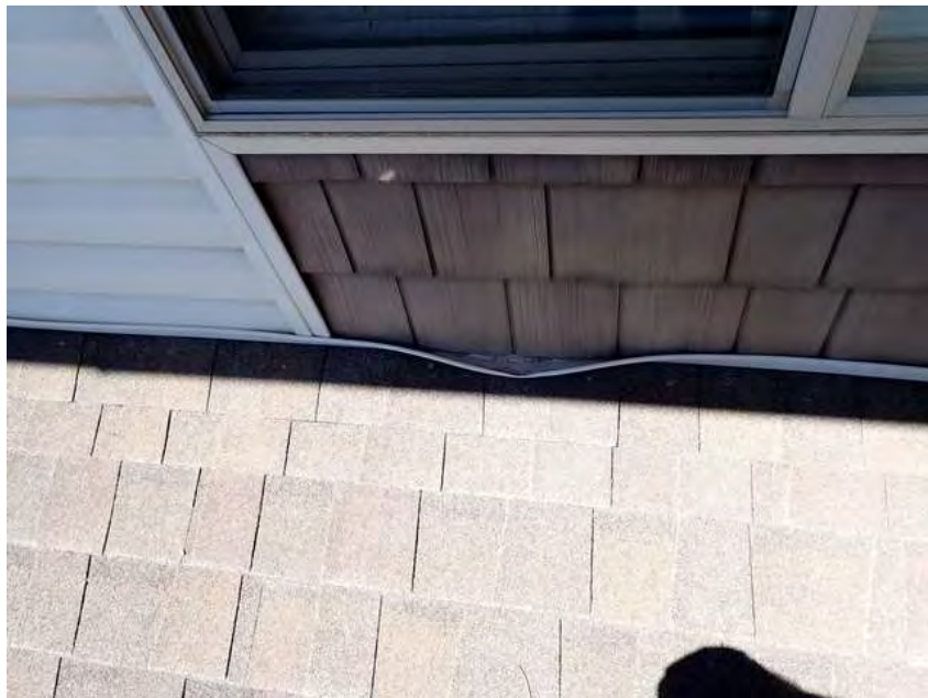
136. Building 7. Deformation in trim.
