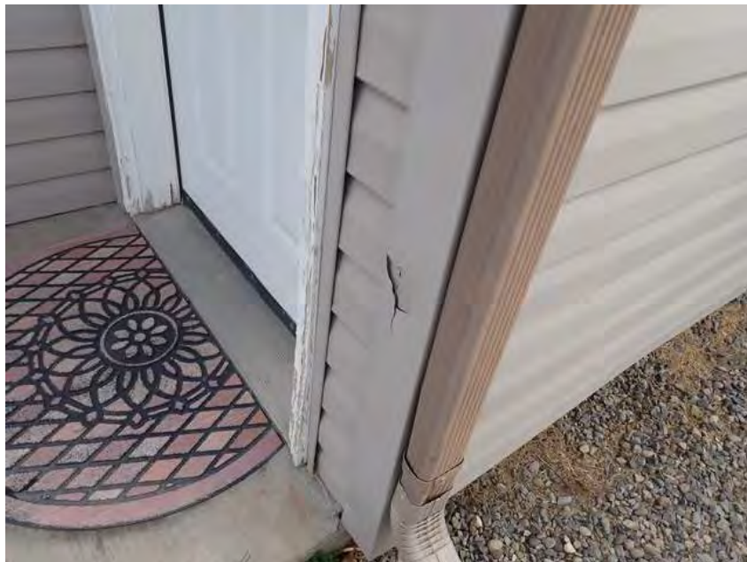
94. Building 6 Fractured siding.
