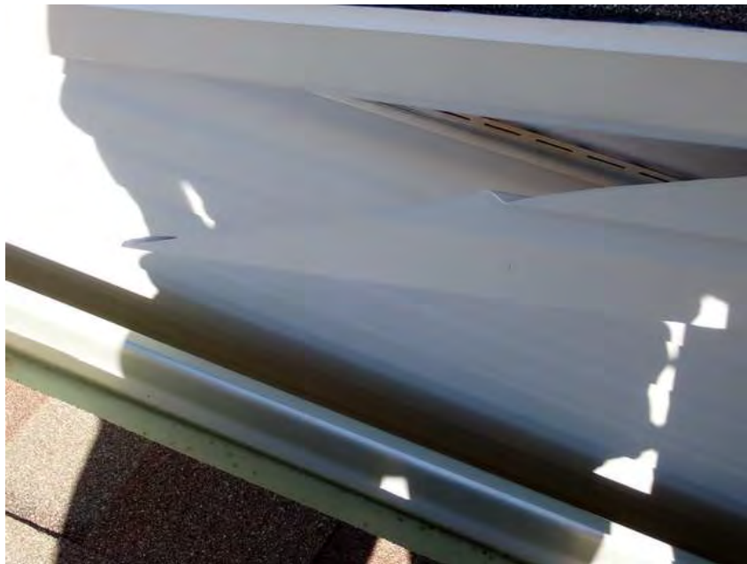
374. Building 22. Displaced siding.
