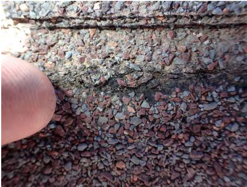
387. Building 22. Detail of crease.
