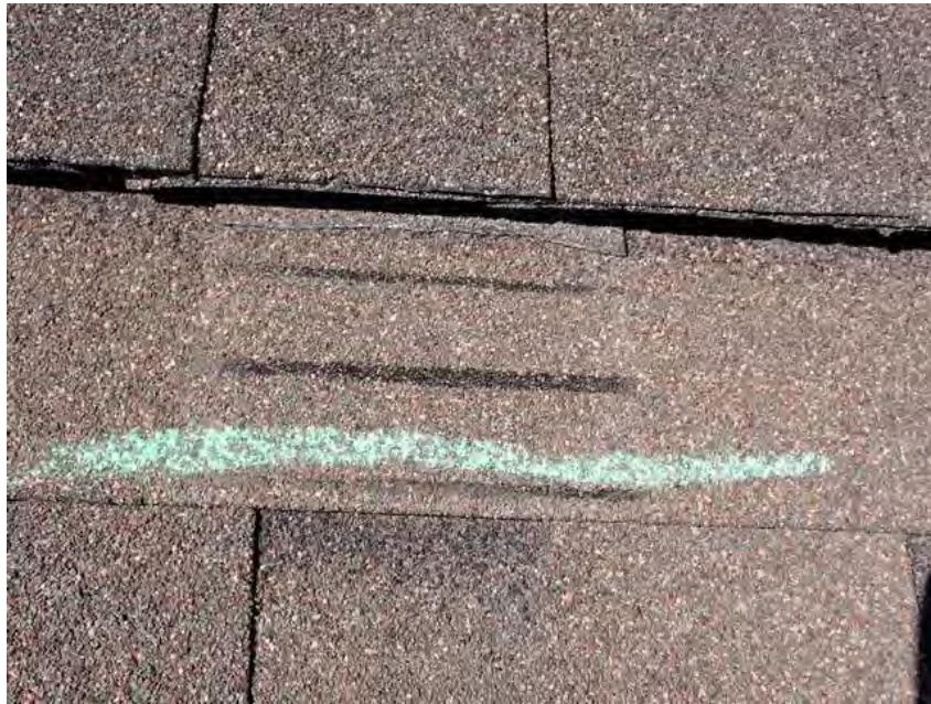
389. Building 22. Missing tooth on shingle.
