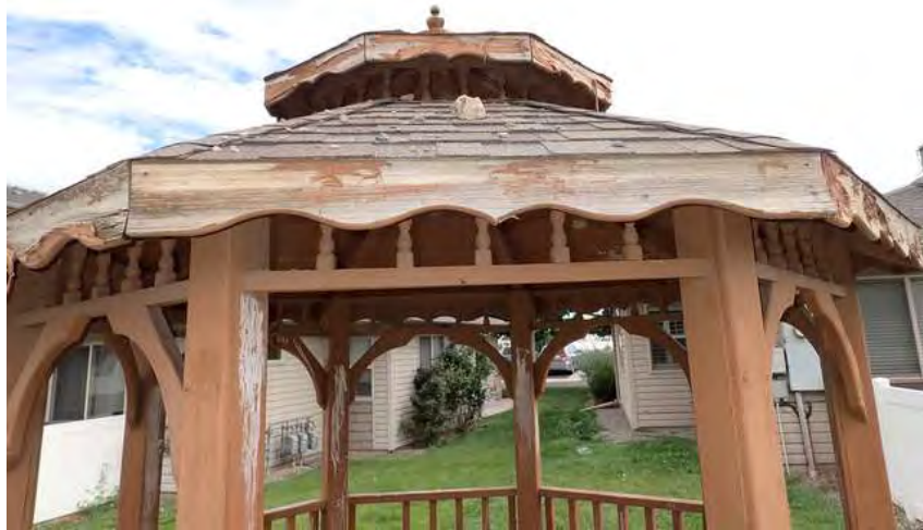
73. Building 4. Gazebo 1 had asphalt shingles. Rocks have been thrown on the roof of gazebo 1.
