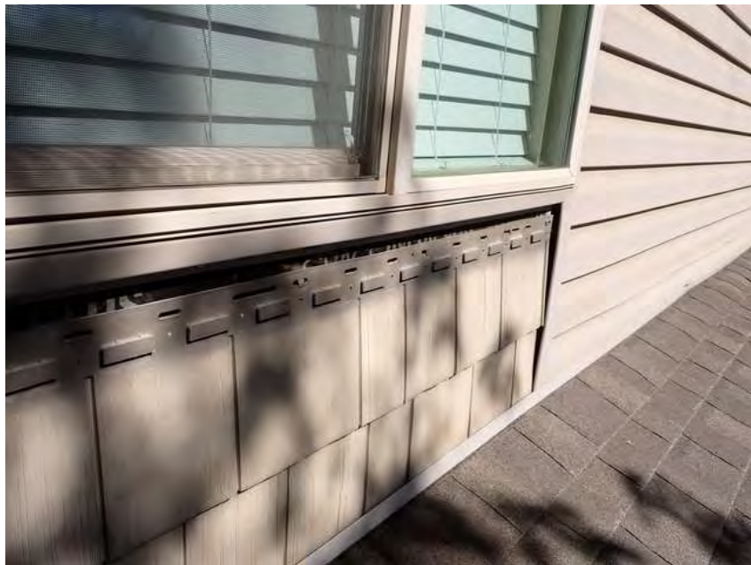
38. Building 2. Detail of missing trim.
