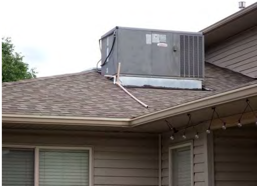
77. Building 5. PVC drainage pipe from AC unit not secured to roof.
