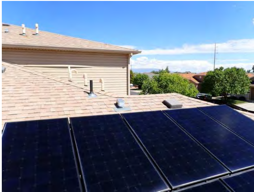
405. Building 23. Solar panels.
