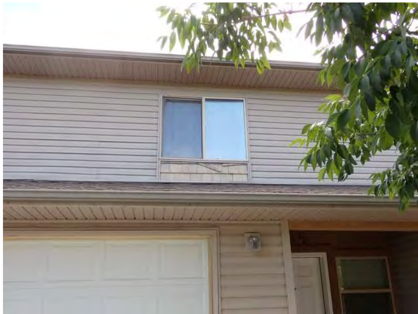
142. Building 8. Sagged vinyl shakes.
