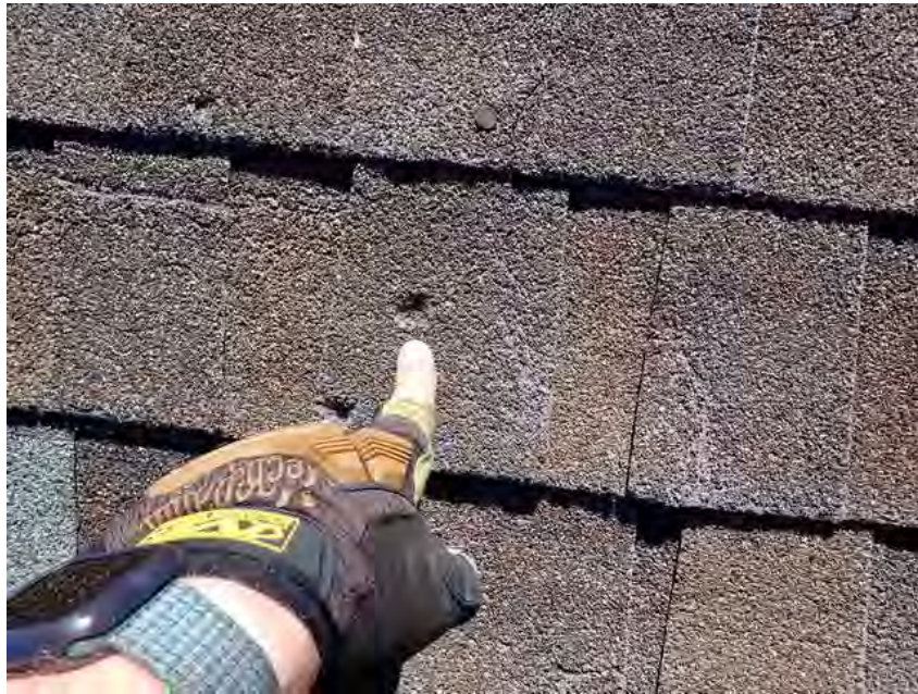
21. Building 1. Puncture in shingle.
