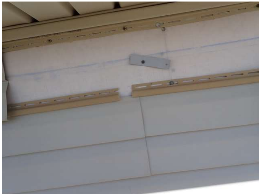
370. Building 22. Missing siding.
