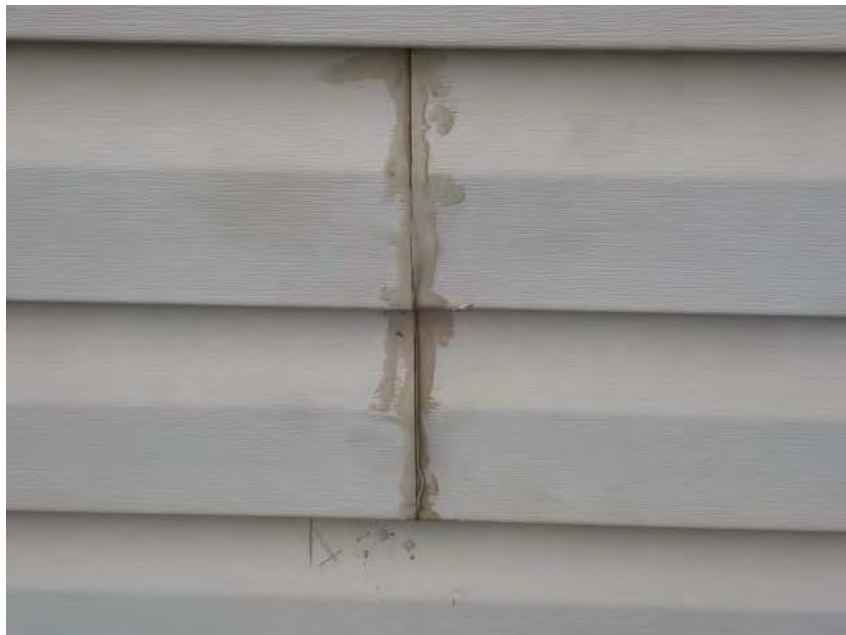
34. Building 2. Patched gap in siding.
