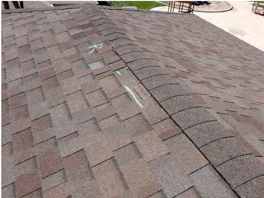
388. Building 22. Missing tooth on shingle.
