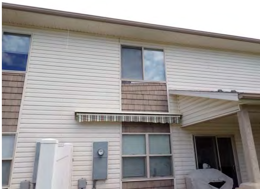
128. Building 7. Sagged vinyl shakes.
