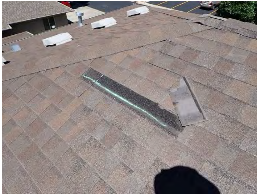
109. Building 6 Missing shingle due to recent winds.
