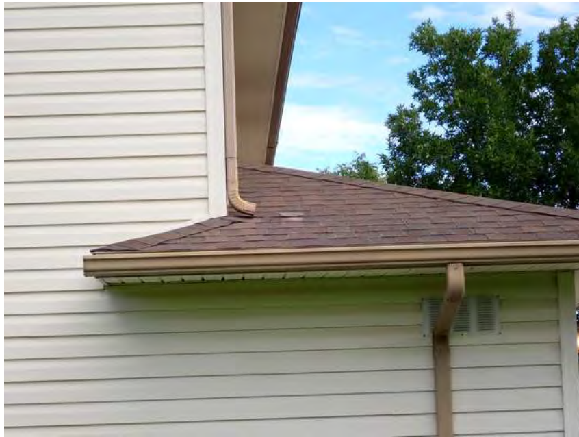
131. Building 7. Shingle tooth flipped back, possible due to downspout proximity.
