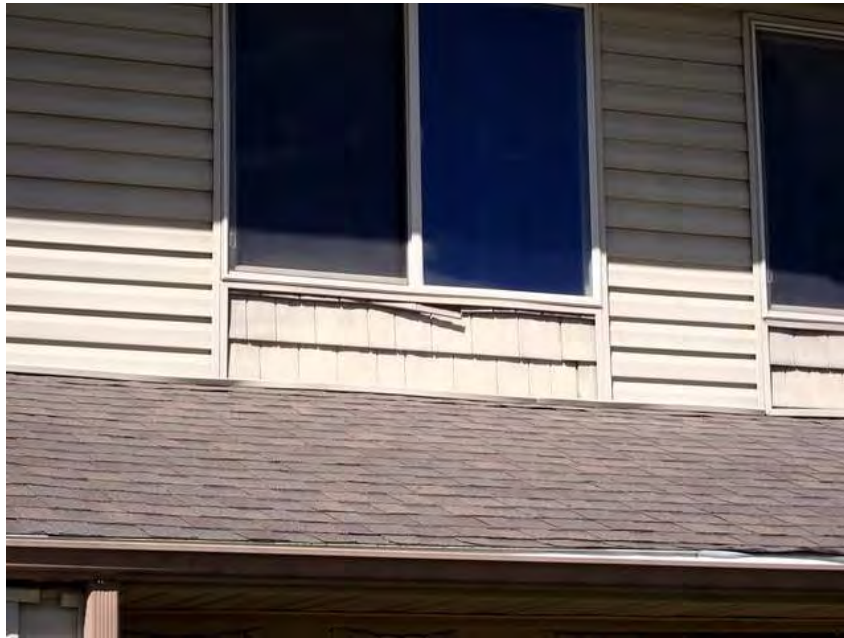
161. Building 9. Sagged vinyl shakes.
