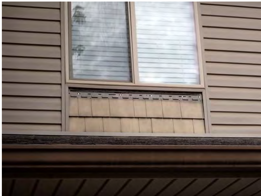
30. Building 2. Missing trim over vinyl shakes.
