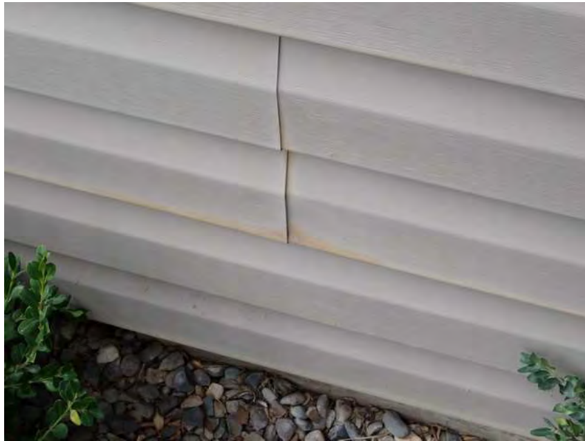
33. Building 2. Discoloration on vinyl siding.
