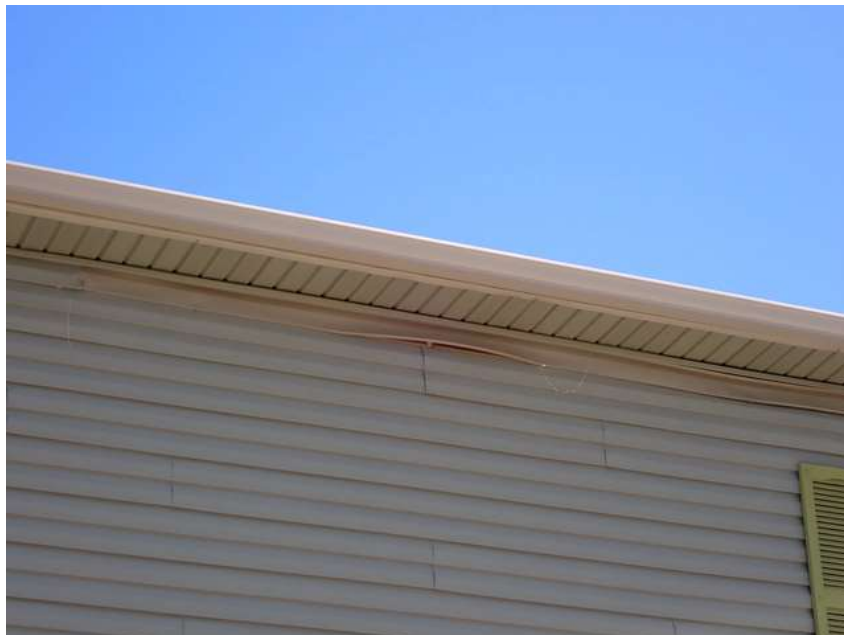
334. Building 20. Deformation in siding.
