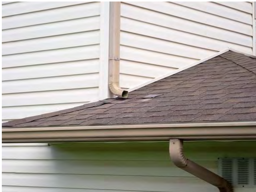
132. Building 7. Shingle tooth flipped back, possible due to downspout proximity.
