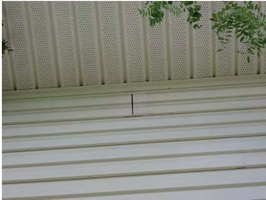
127. Building 7. Gap in siding.
