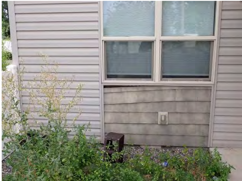
36. Building 2. Sagged vinyl shakes.
