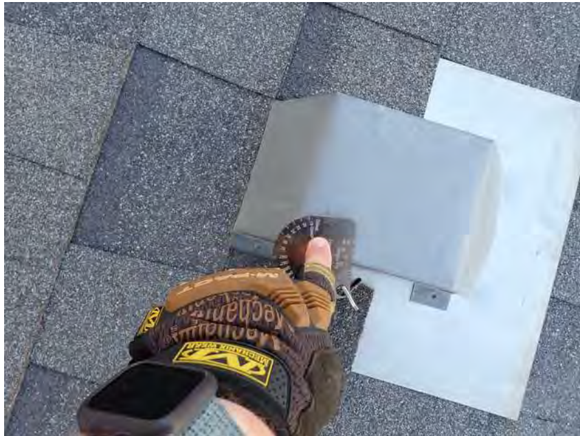
423. Building 24. Dryer vents made from steel.
