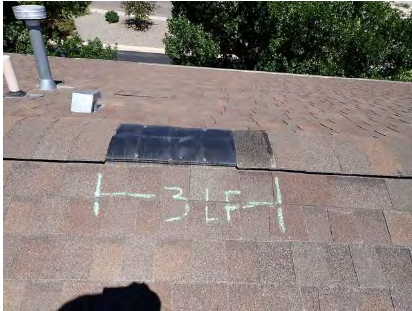
121. Building 6 Missing ridge cap.
