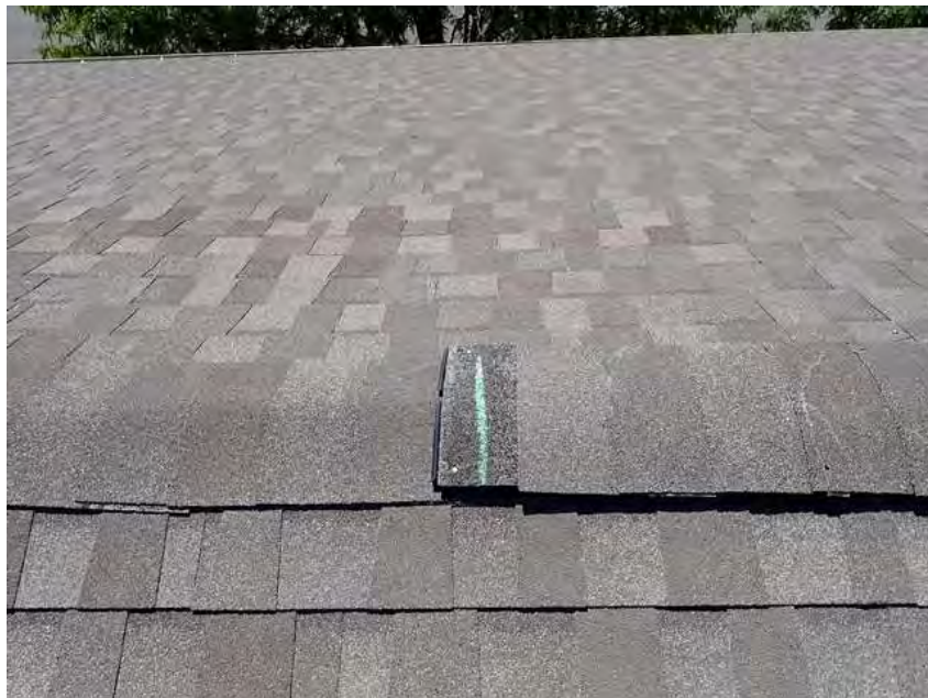
194. Building 11. Missing ridge cap.
