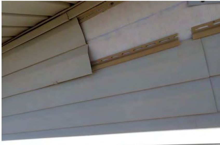
371. Building 22. Missing siding.
