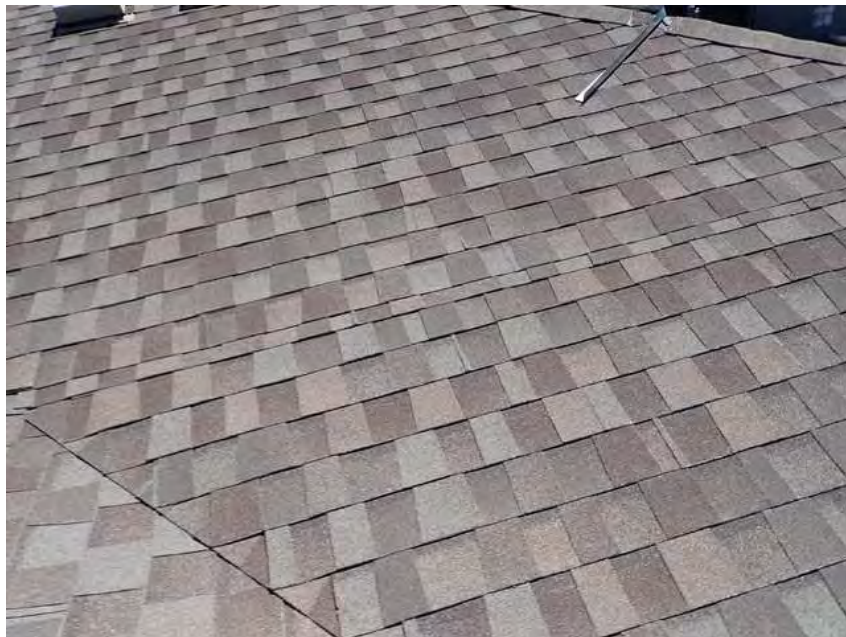
84. Building 5. Shingle misalignment.
