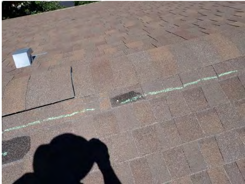
120. Building 6 Torn shingle.
