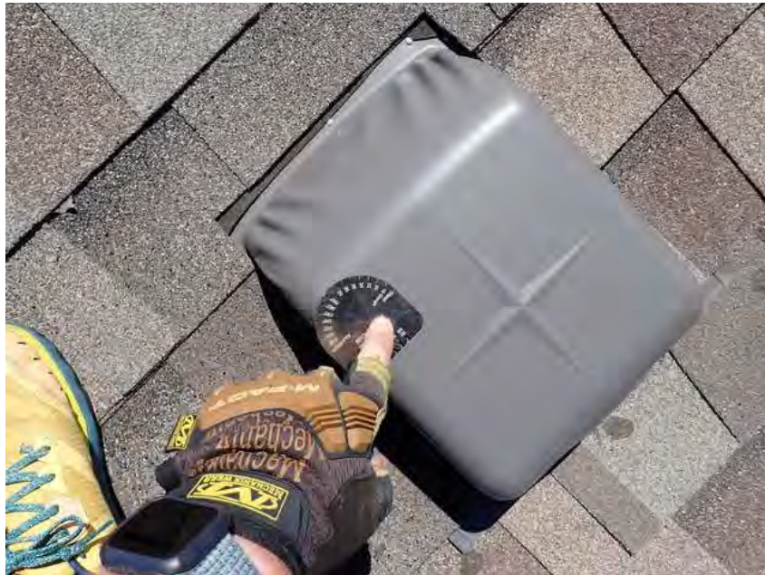
89. Building 5. Steel vent boxes on this building.
