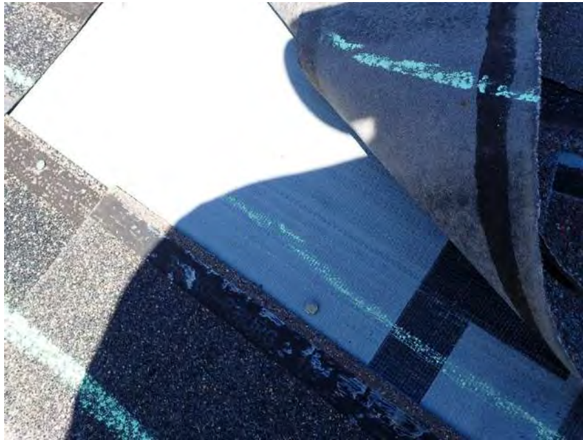
115. Building 6 Roof barrier exposed.
