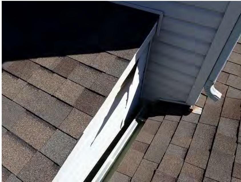
373. Building 22. Displaced siding.
