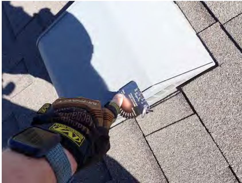
331. Building 19. Steel vent boxes on this building.
