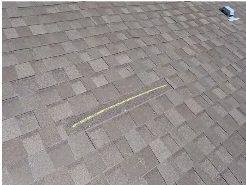
192. Building 11. Missing shingle.
