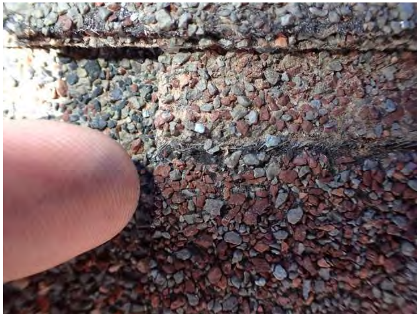
386. Building 22. Detail of crease.
