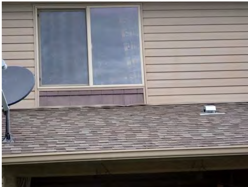
78. Building 5. Deformation of trim.
