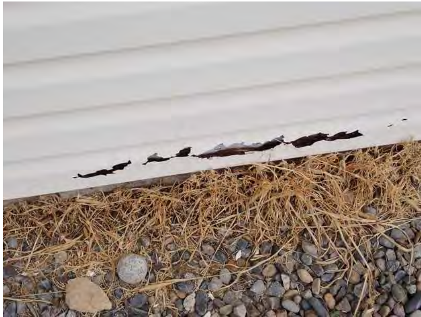
45. Building 3. Tear in vinyl siding. Likely mechanical damage from string trimmer.
