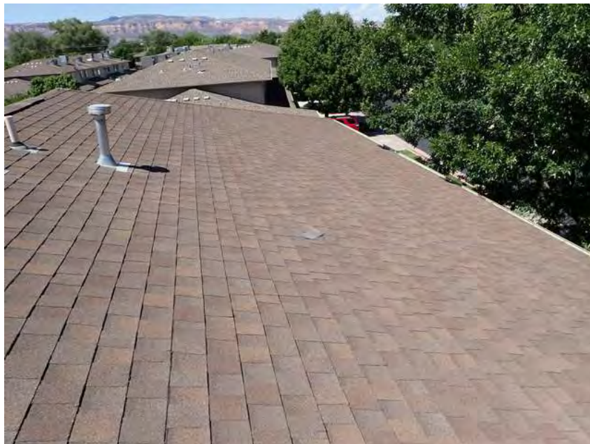
106. Building 6 Loose shingle fragment.
