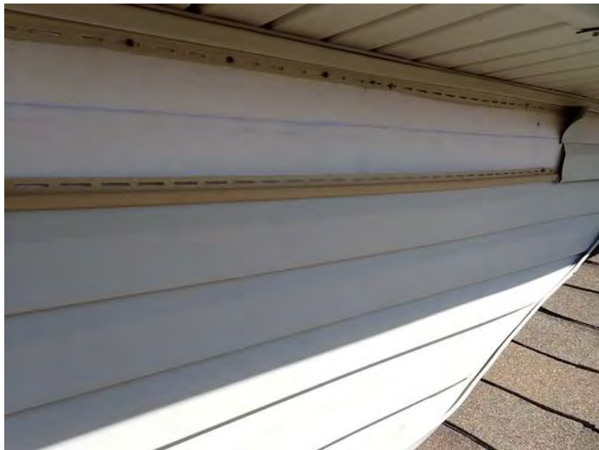
372. Building 22. Missing siding.
