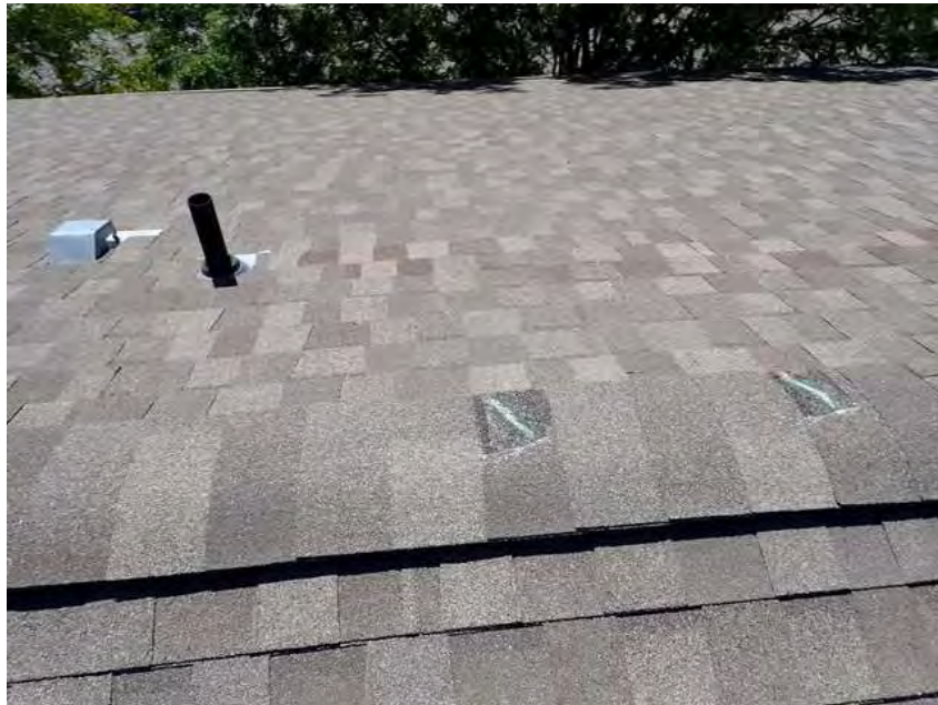
195. Building 11. Torn ridge caps.
