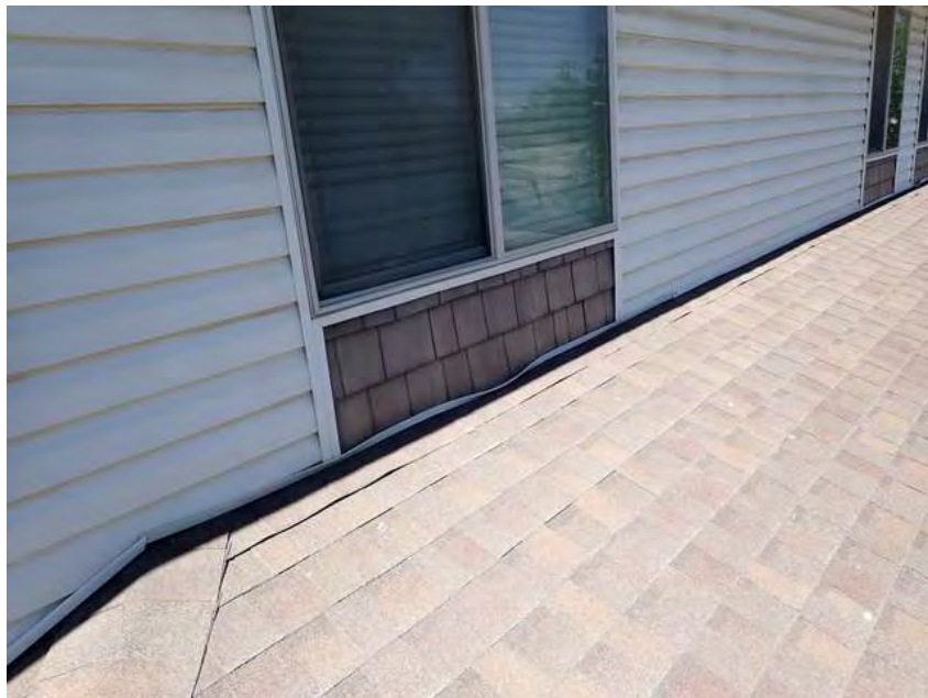
134. Building 7. Deformation in trim.
