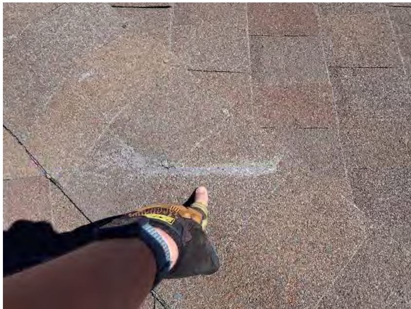
16. Building 1. Detail of mechanical impact.
