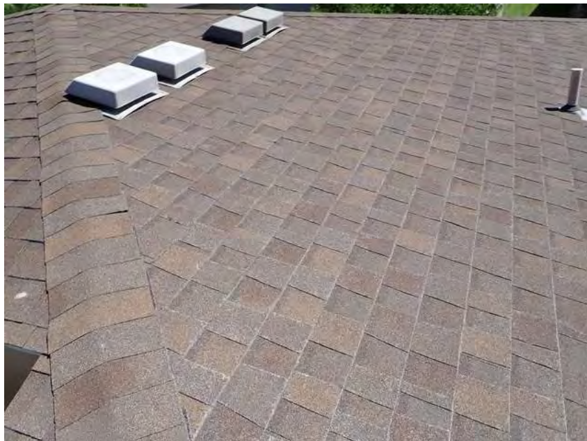
138. Building 7. Weathering on shingles.
