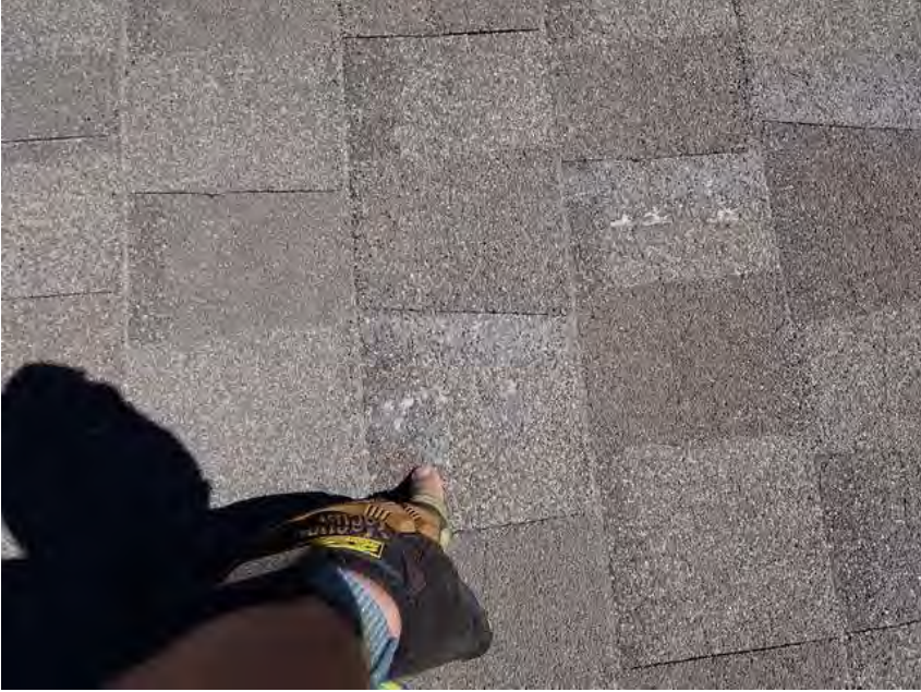
41. Building 2. Granule loss.
