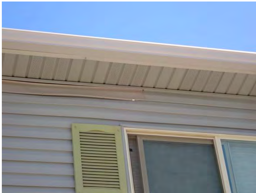
336. Building 20. Deformation in siding.
