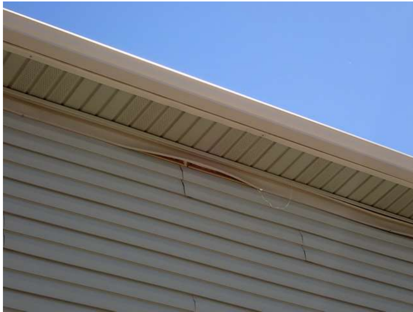
335. Building 20. Deformation in siding.
