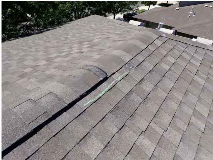
196. Building 11. Missing shingle.
