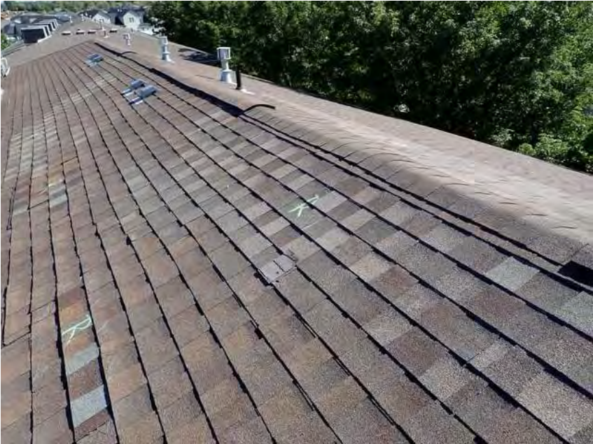
20. Building 1. Multiple repairs.
