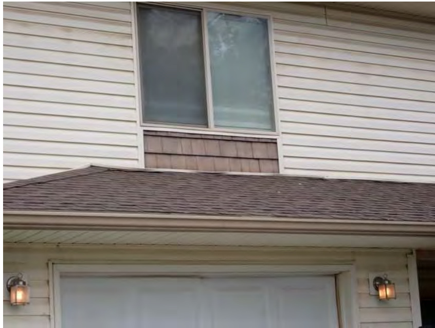
125. Building 7. Deformation in trim.
