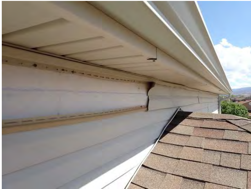
369. Building 22. Missing siding.
