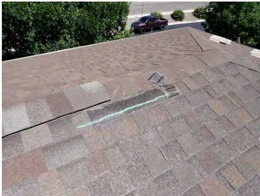
122. Building 6 Missing shingle.
