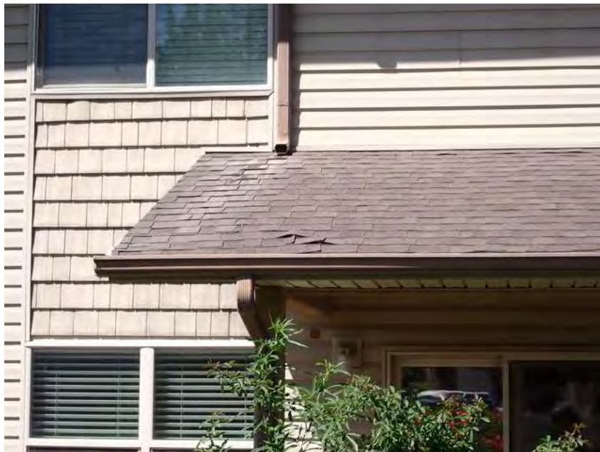
160. Building 9. Puckered shingles likely from underdriven fasteners.
