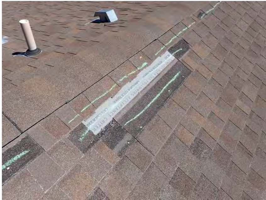
119. Building 6 Missing shingles from recent winds.
