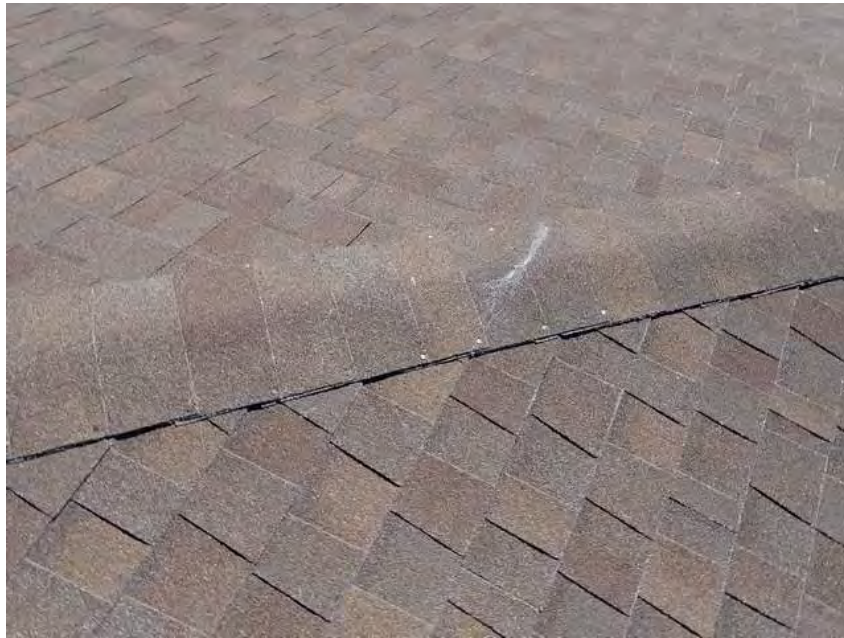
15. Building 1. Mechanical impact to ridge cap shingles.
