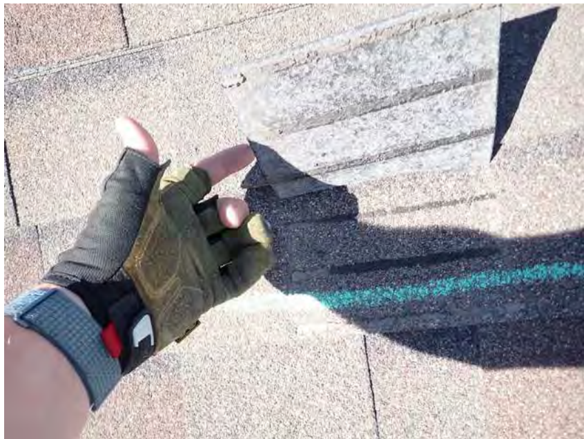
384. Building 22. Creased tooth on shingle.
