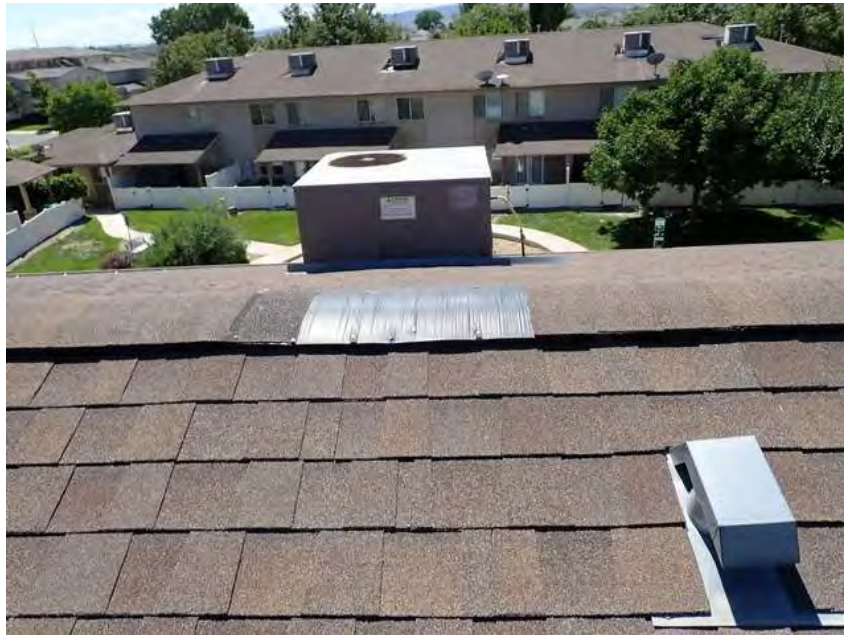
105. Building 6 Missing shingles from ridge cap.
