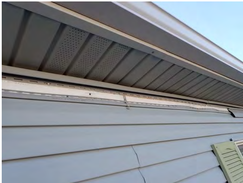
348. Building 20. Missing siding.
