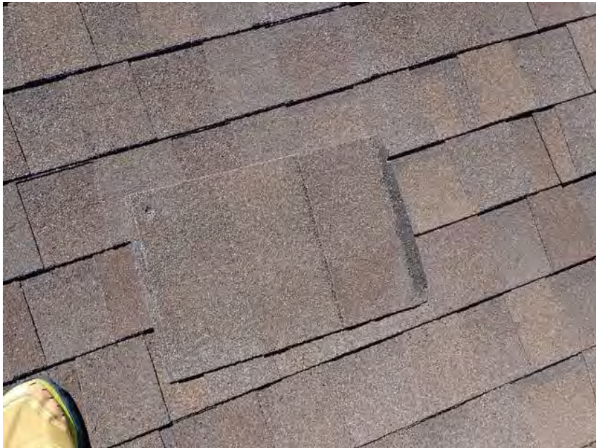
104. Building 6 Loose ridge cap shingle found on roof field.
