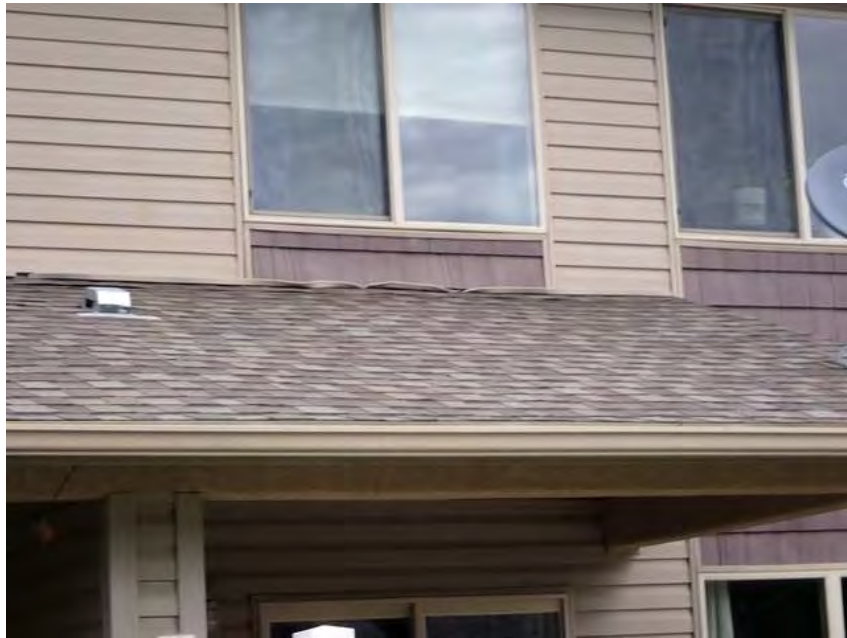
79. Building 5. Deformation of trim.
