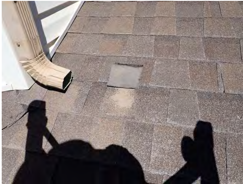
133. Building 7. Shingle tooth flipped back, possible due to downspout proximity.
