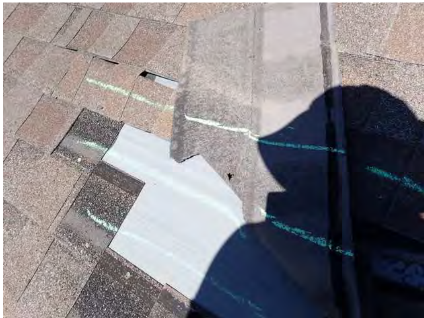
116. Building 6 Adjacent shingles appear to have slipped.
