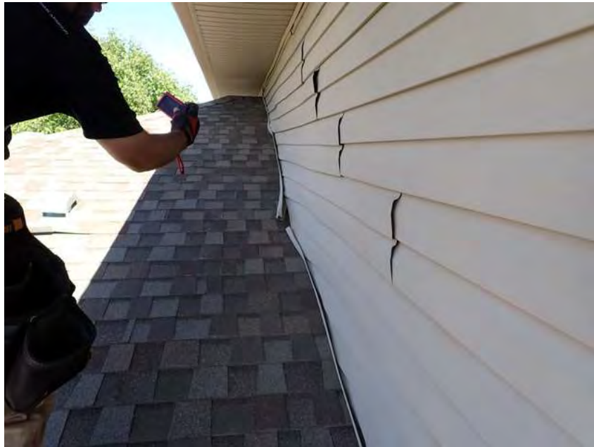
85. Building 5. Gaps in siding.
